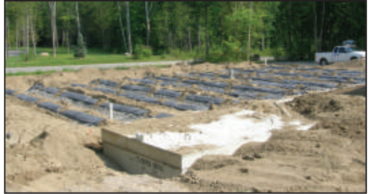
Septic tank and leaching bed.
