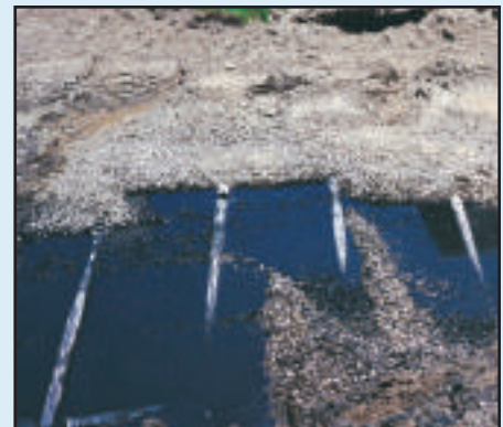
A failed system exposed.
